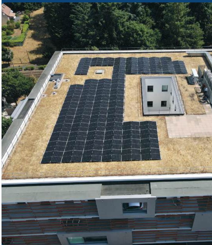
Photovoltaic self-consumption plant installed in May 2025 on the roof of our headquarters, Obeya.
